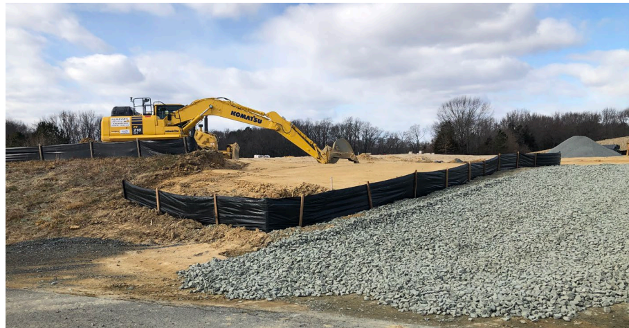
An active construction site using silt fence and a stabilized construction entrance in order to reduce surface runoff from the project
